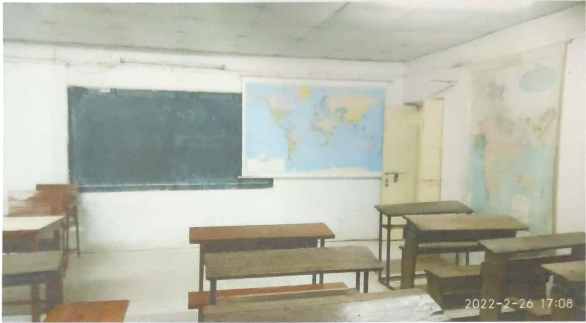
Photo 14 Well tube light facility in Classroom
